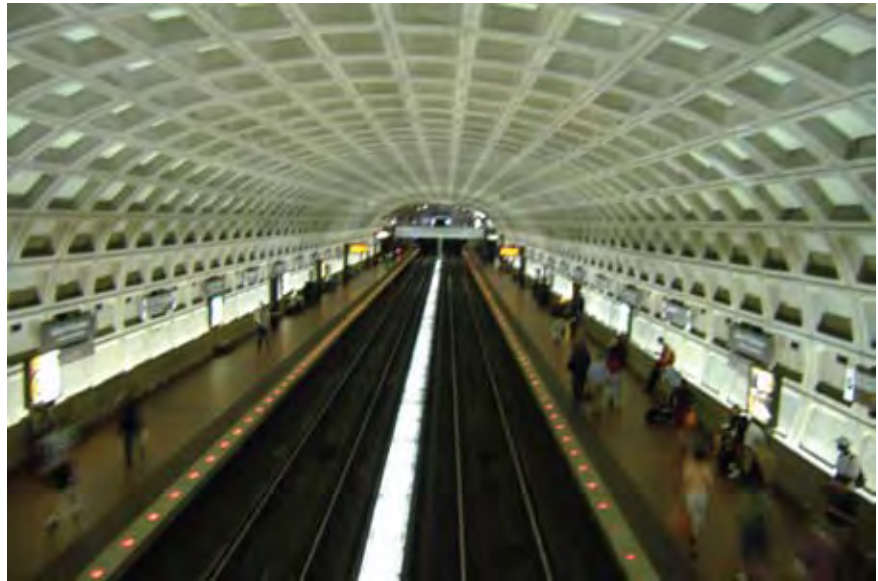
The vaulted ceilings create the intended effect: this is a substantial system.
