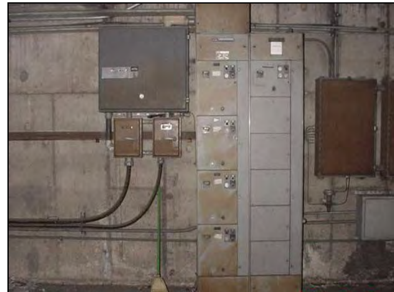
Motor Control Center
