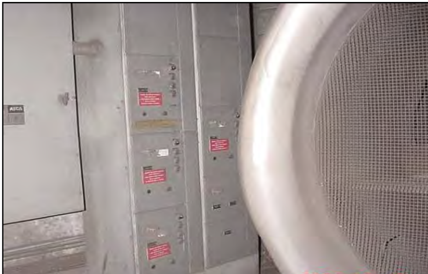
Serves Ventilation Fans & Drainage Pumps
