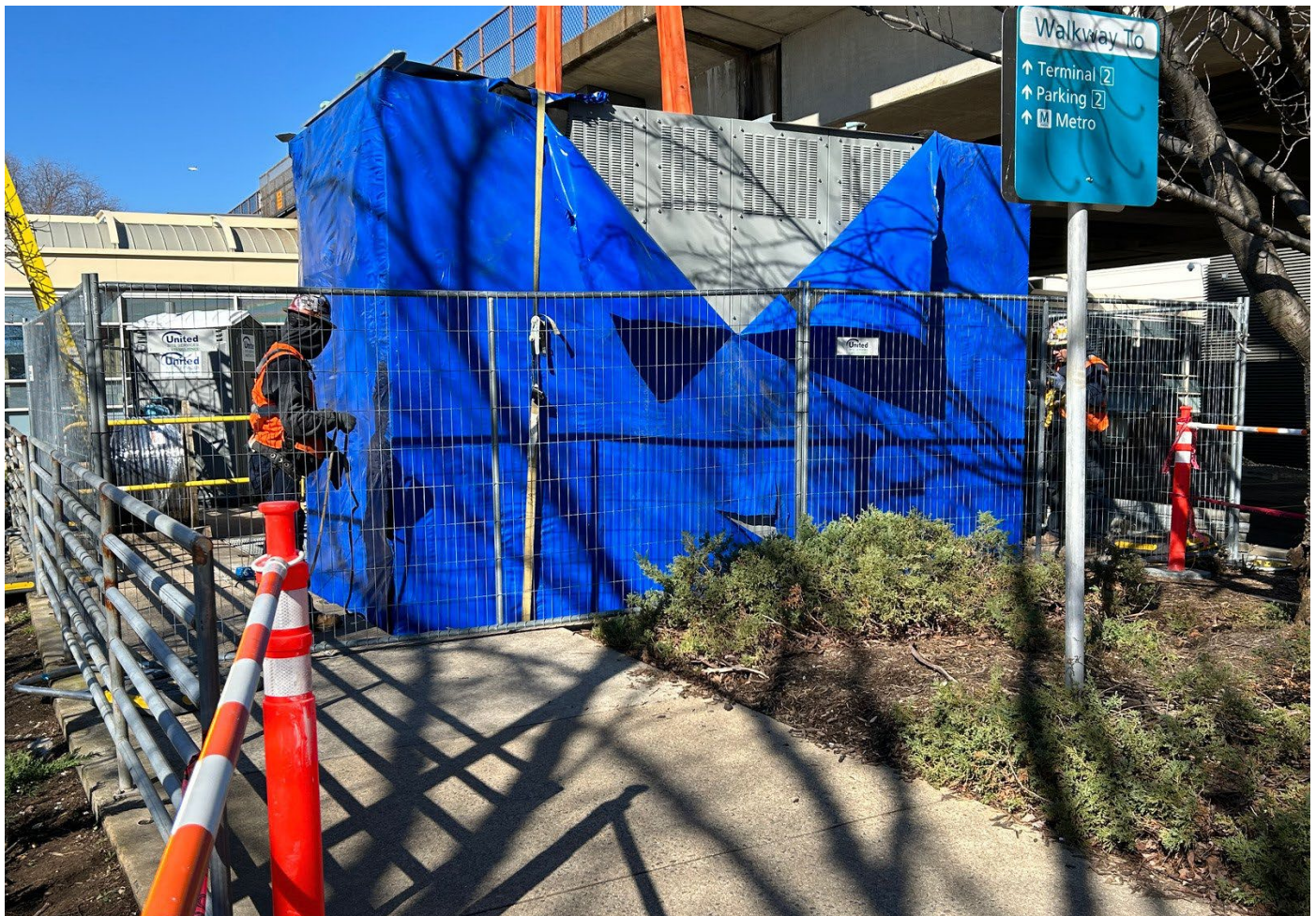
Metrorail traction power upgrade on Blue and Yellow line in preparation for Potomac Yard station
